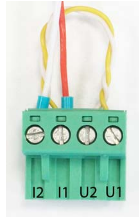
connected 2 wire Pt 100
